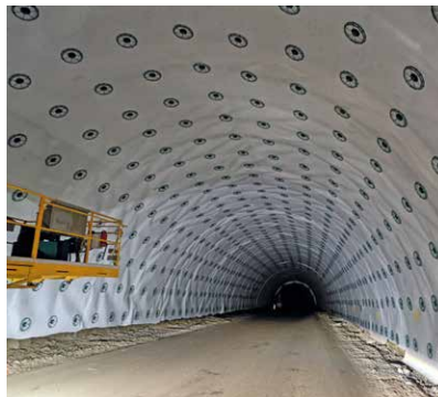
The spacers in the construction of the Sandoy tunnel in the Faroe Islands.
