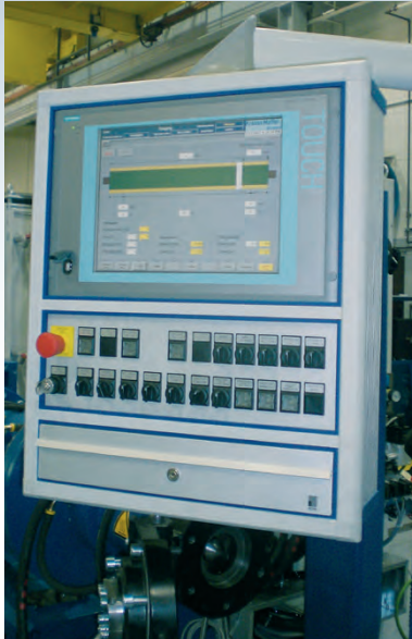
Central operator panel
